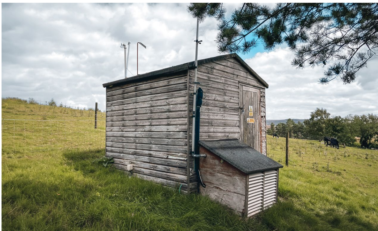
Figure 6: Ladybower current cabin, due for replacement.
